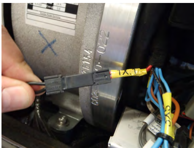
Fig. 15.5-1: Not Stop bridge in the cable harness
