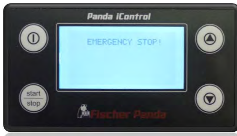
Fig. 15.5-2: Panel shows Emergency Stop
