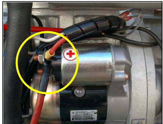
Fig. 6.11.2-1: Positive Battery Cable
