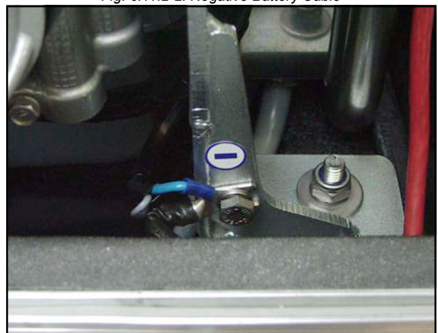
Fig. 6.11.2-2: Negative Battery Cable
