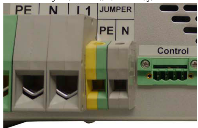
Fig. 11.5.1.4-1: External PE/N Bridge
